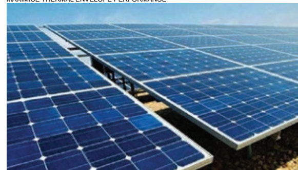
ROOFTOP PV ARRAYS
